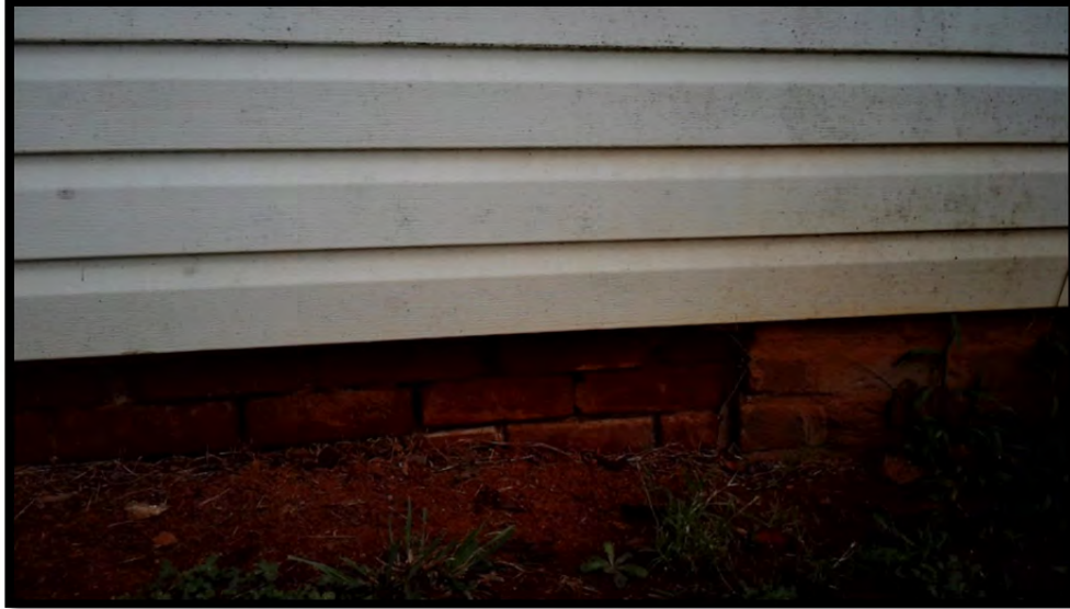
Vinyl siding over wood; disintegrated mortar joints in foundation
